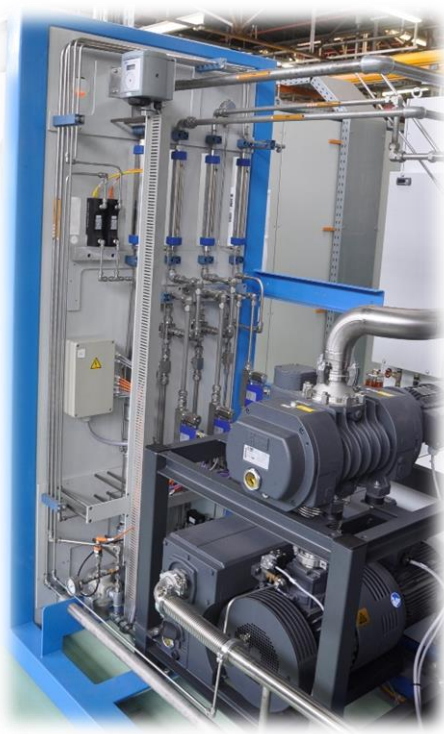
Gas panel with vacuum pump
